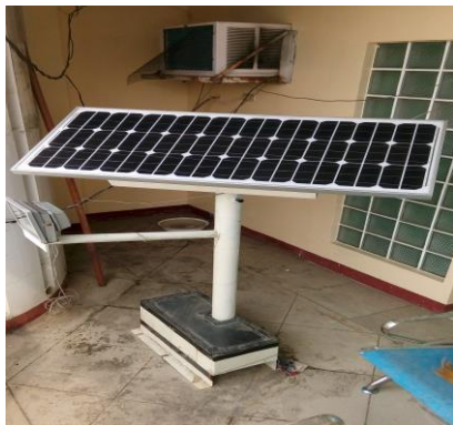
Fig. 2. Solar Lighting System 1 & 2
