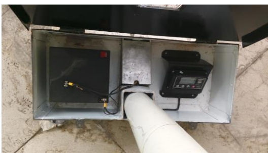
Fig. 3. Solar battery 26Amps and controller 10Amps
